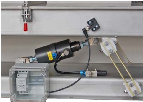
Vibration monitoring system at conveyor with blade springs
